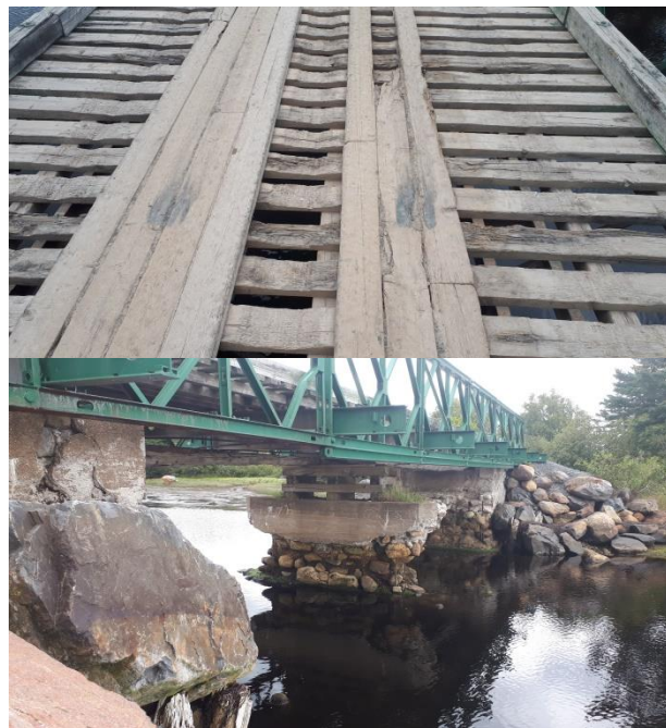
Bridge at the 4.0km mark. Notice the worn decking that needs immediate attention.
