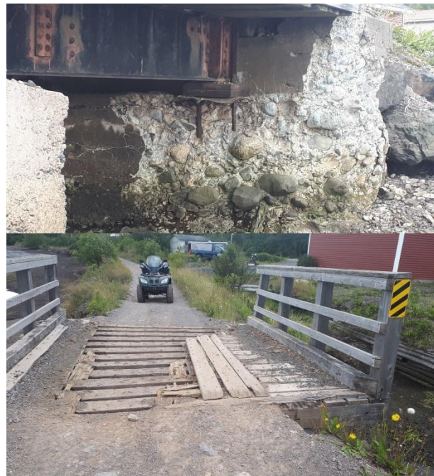
This bridge requires significant repairs.
